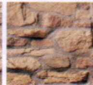
Wide Mortar Joints, Overgrout
